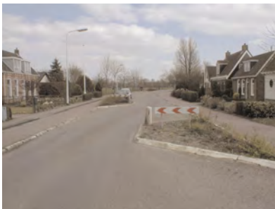
Poorly designed traffic calming.
